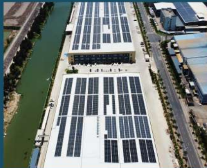
Taizhou 6.8MWp Distributed Solar Power Plant
