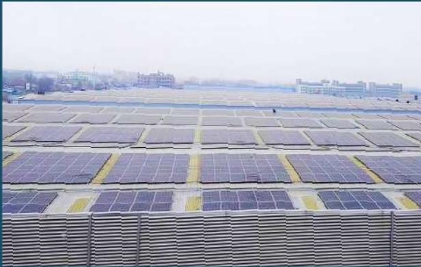
Xinzheng 6.2MWp Distributed Solar Power Plant
