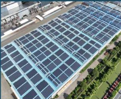
Taizhou 5.537MWp Distributed Solar Power Plant
