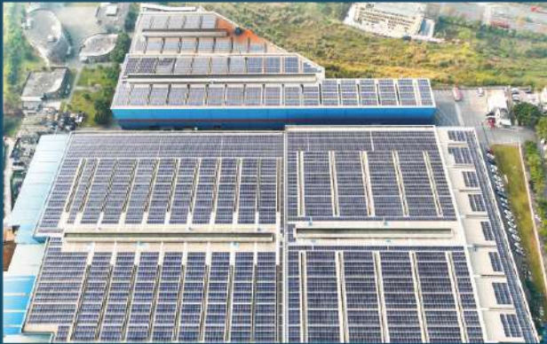
Chongqing 5.6MWp Distributed Solar Power Plant
