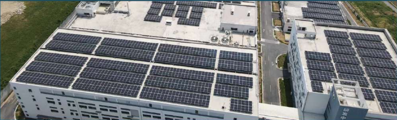
Anhui 1.98MWp Distributed Solar Power Plant
