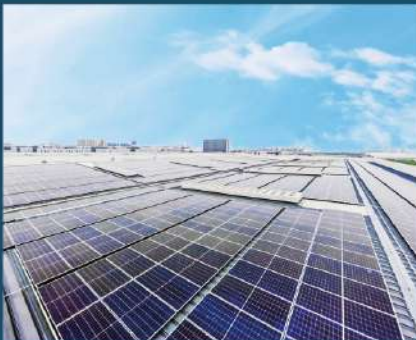
Hangzhou 6.73MWp Distributed Solar Power Plant
