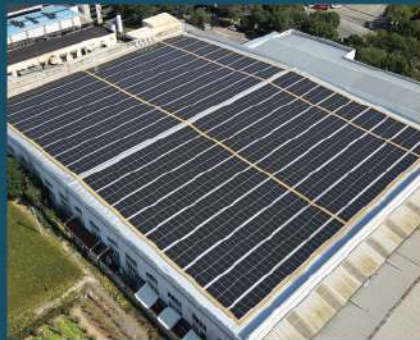
Ningbo 1.68MWp Distributed Solar Power Plant
